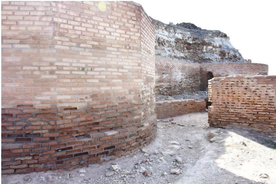
Erosion of the bricks in the tower of the inner wall of the castle
