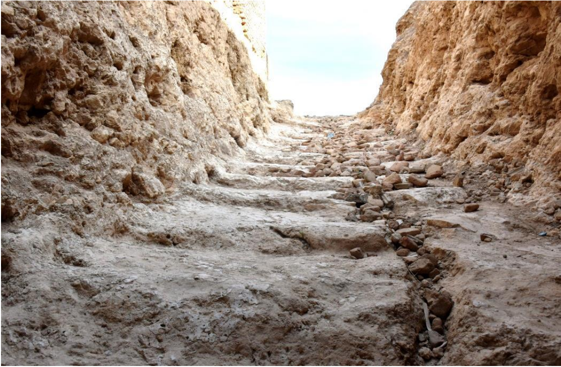
Corrosion in the staircase of the access tunnel to the roof of the castle
