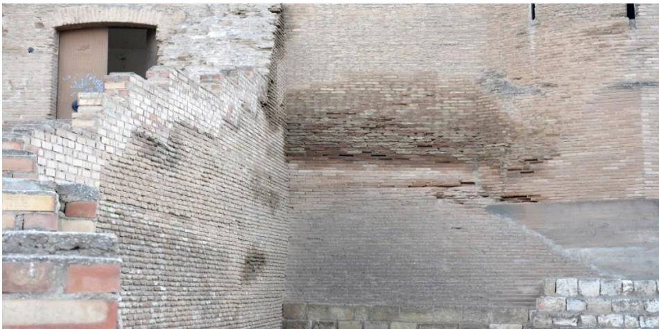
Damage at point 1 of the outer wall to the right of the main gate
