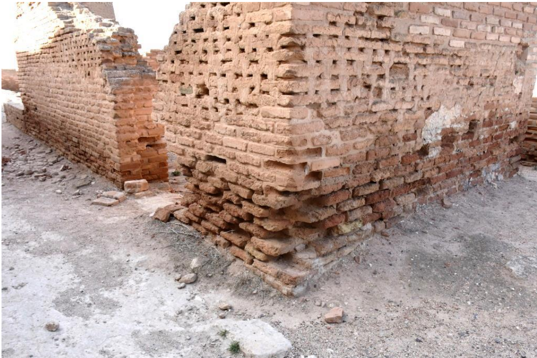
Brick erosion in the corner of buildings attached to the towers of the outer wall
