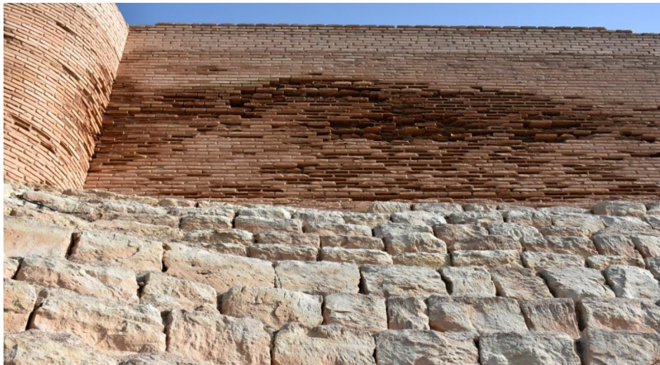
Damage at point 4 of the outer wall
