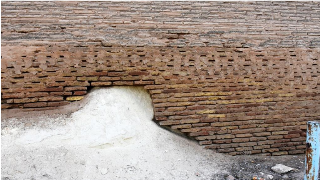
Moisture at the bottom of the wall from the first tower to the fourth tower is eroding the bond between the bricks
