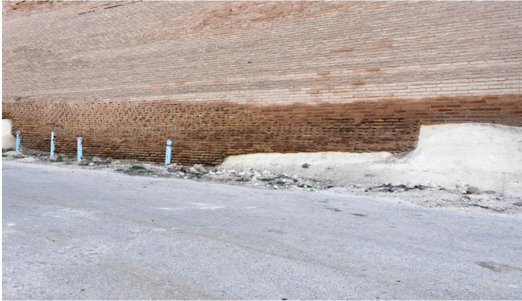
Humidity in the face down the wall and towers from the first to the fourth towers of the outer wall
