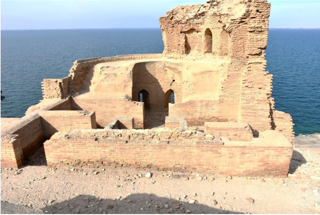
General view of one of the towers of the inner wall of the castle T5
