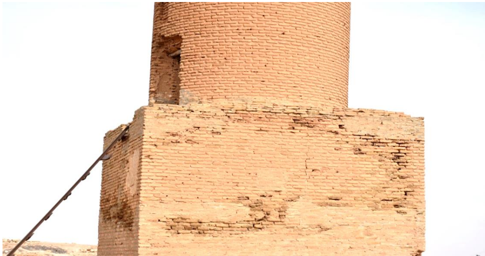
Erosion in the bricks and plaster
