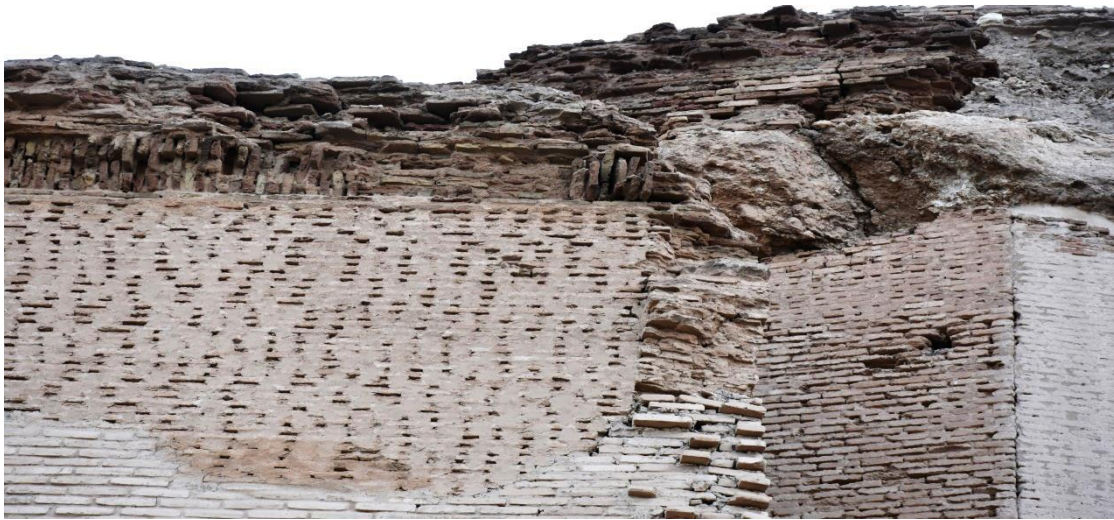
Damage point of the outer wall from the emirate Tower to the first tower
