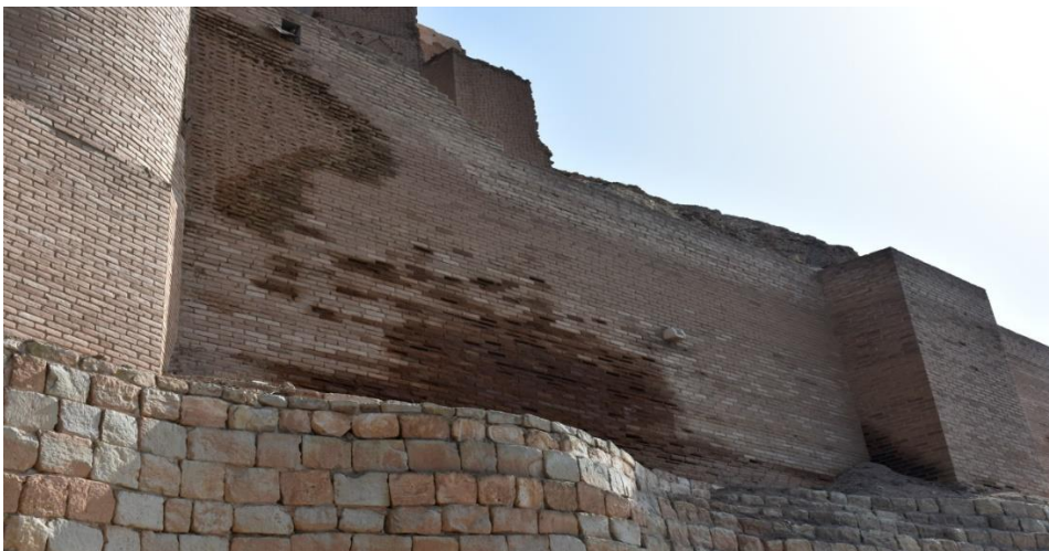
Damage at point 2 of the outer wall to the right of the main gate overlooking the river
