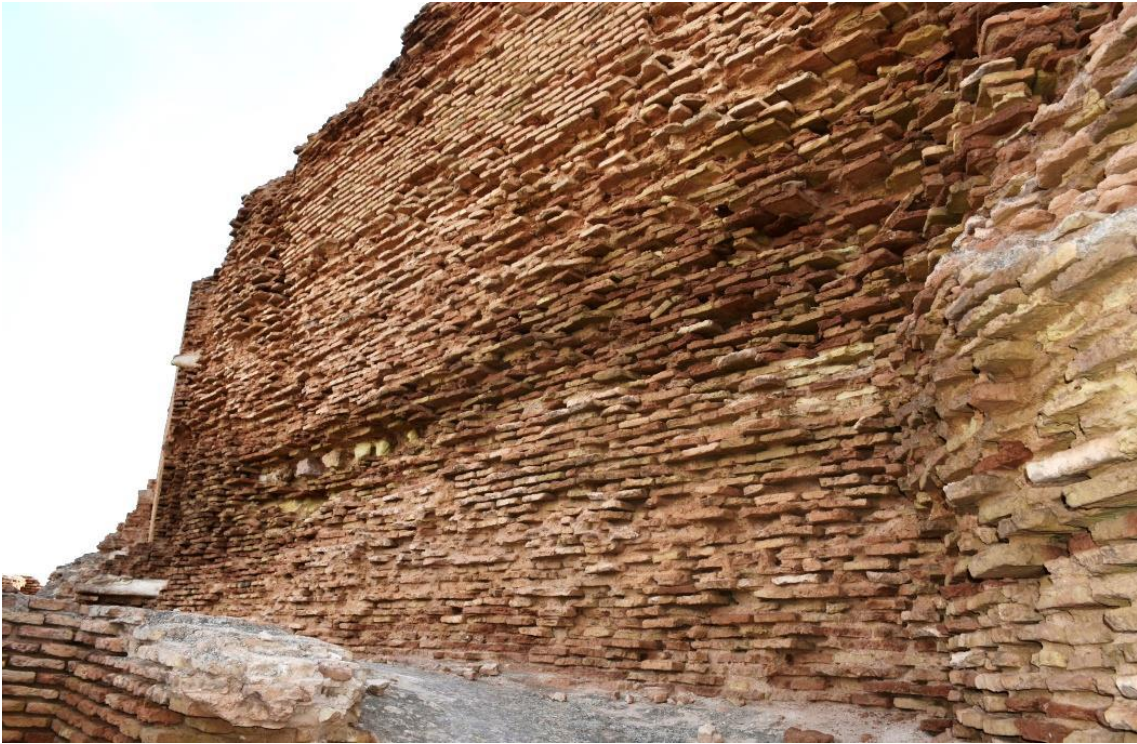
Loss of brick in one of the walls of the inner wall.
