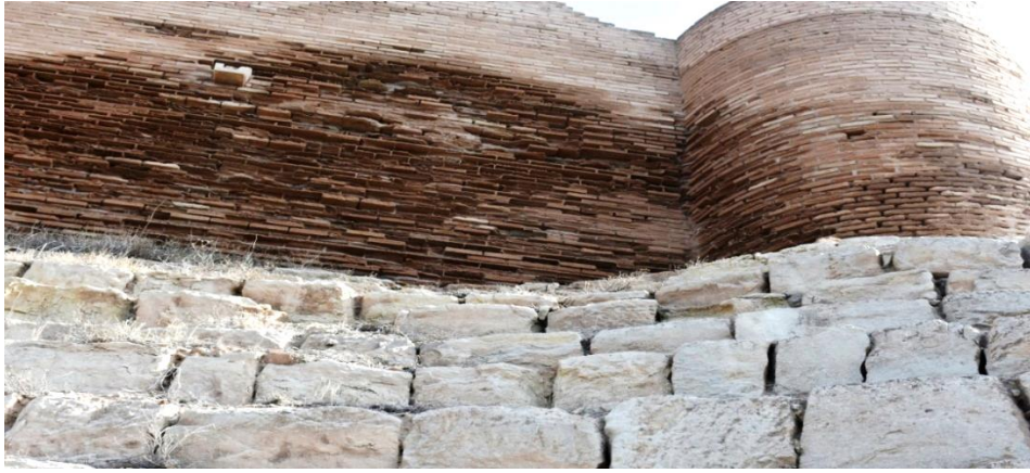
Damage at point 3 of the outer wall
