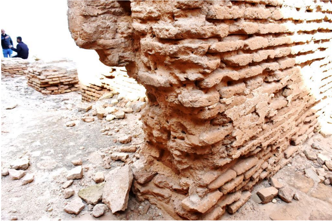
Corrosion and loss of bricks in the buildings attached to the towers of the outer wall
